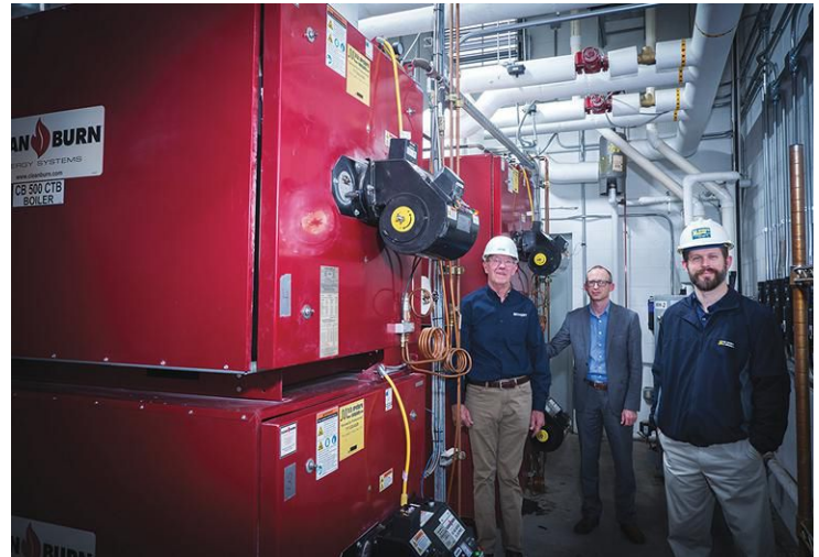
From left, Howe, Knaub and Shamenek stand beside Clean Burn CB500 boilers. Bell & Gossett pumps are installed above their heads.
