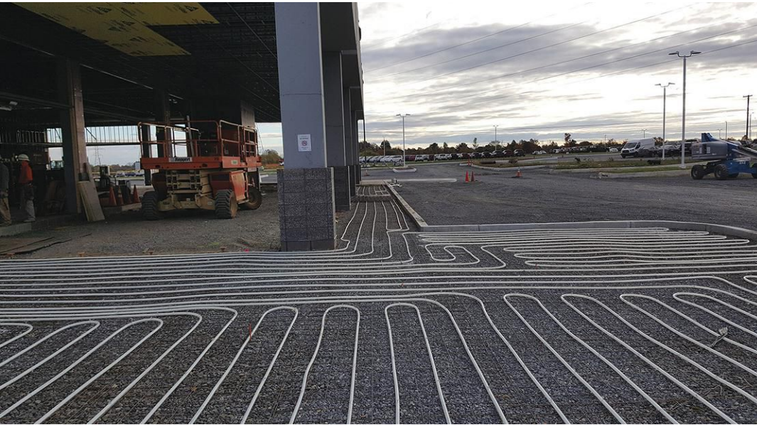
The dealership features Uponor Wirsbo hePEX piping for the in-slab snowmelt system at the front entrance and sidewalks, near the showroom canopy (in background). PEX piping is fastened to the wire mesh prior to concrete pour.
