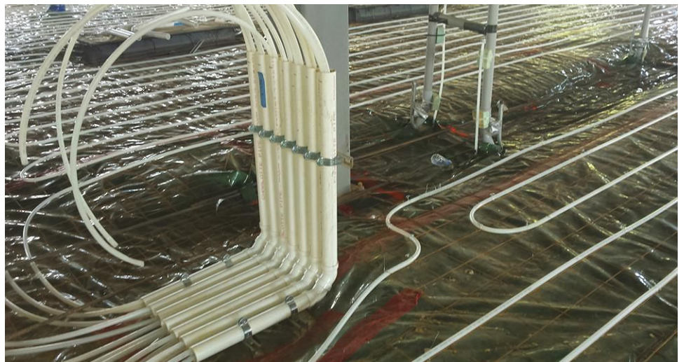
This is the in-slab radiant Uponor Wirsbo hePEX floor piping in the service garage. Shown are 2-inch PVC sleeves for securing and routing the PEX piping below slab, prior to concrete pour.
